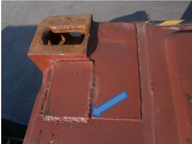
Non-conforming patch exceeds the original size of the Corner Protection Plate.
