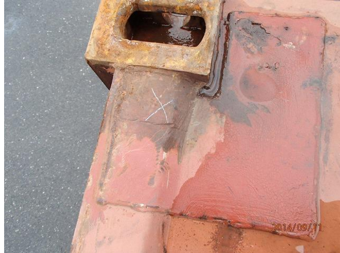
Acceptable insert on corner protection plate. Any damage to the front header must have been repaired prior to insert installation. Repair shall not protrude above the upper face of the corner fitting.
