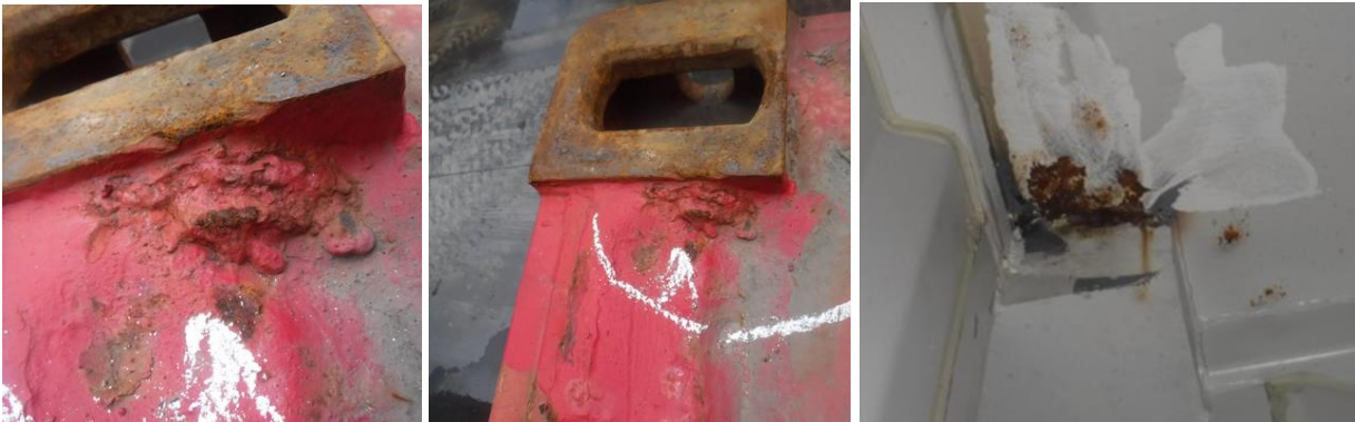
Non-conforming repair. Damaged area filled with weld without restoring original profile of the rear header and corner protection plate.
